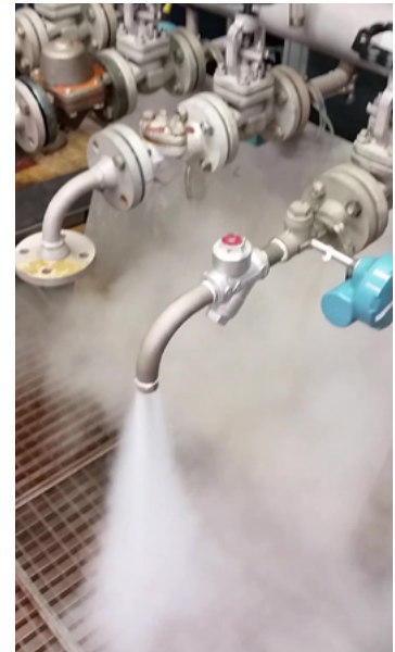
Figure 3: This is not how it should be. Steam escaping from a steam trap (Source: Emerson Automation Solutions) ©Emerson.com
